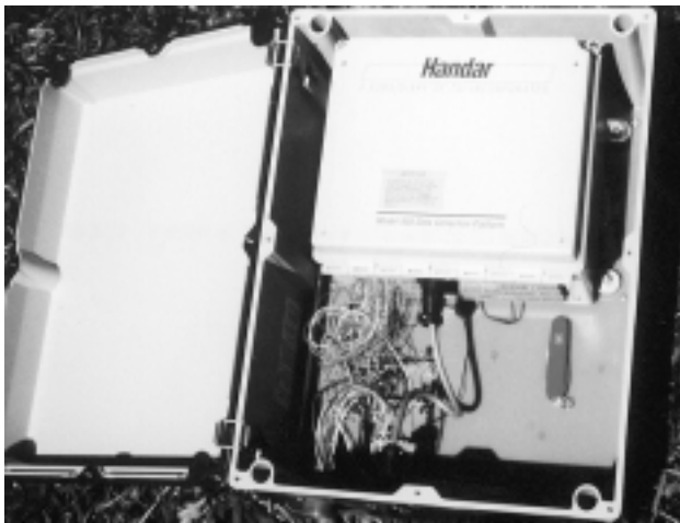
Figure 3—The Handar 555 data-logger is used for auto-logging of thermistor probe readings. Data-logger is shown installed inside a weather-tight utility box.
