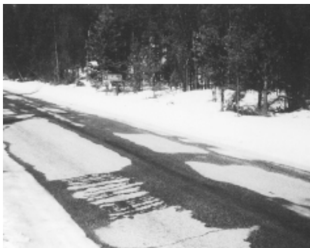
Figure 46—Kootenai National Forest Site 2 on March 14, 1996 near beginning of subsurface thawing. Note the water is “bleeding” up through the pavement.
