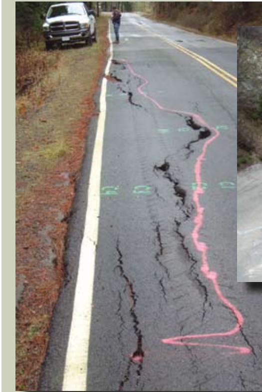
Figure 1—Cracking and settlement along top of slide in asphalt road, Region 6.
