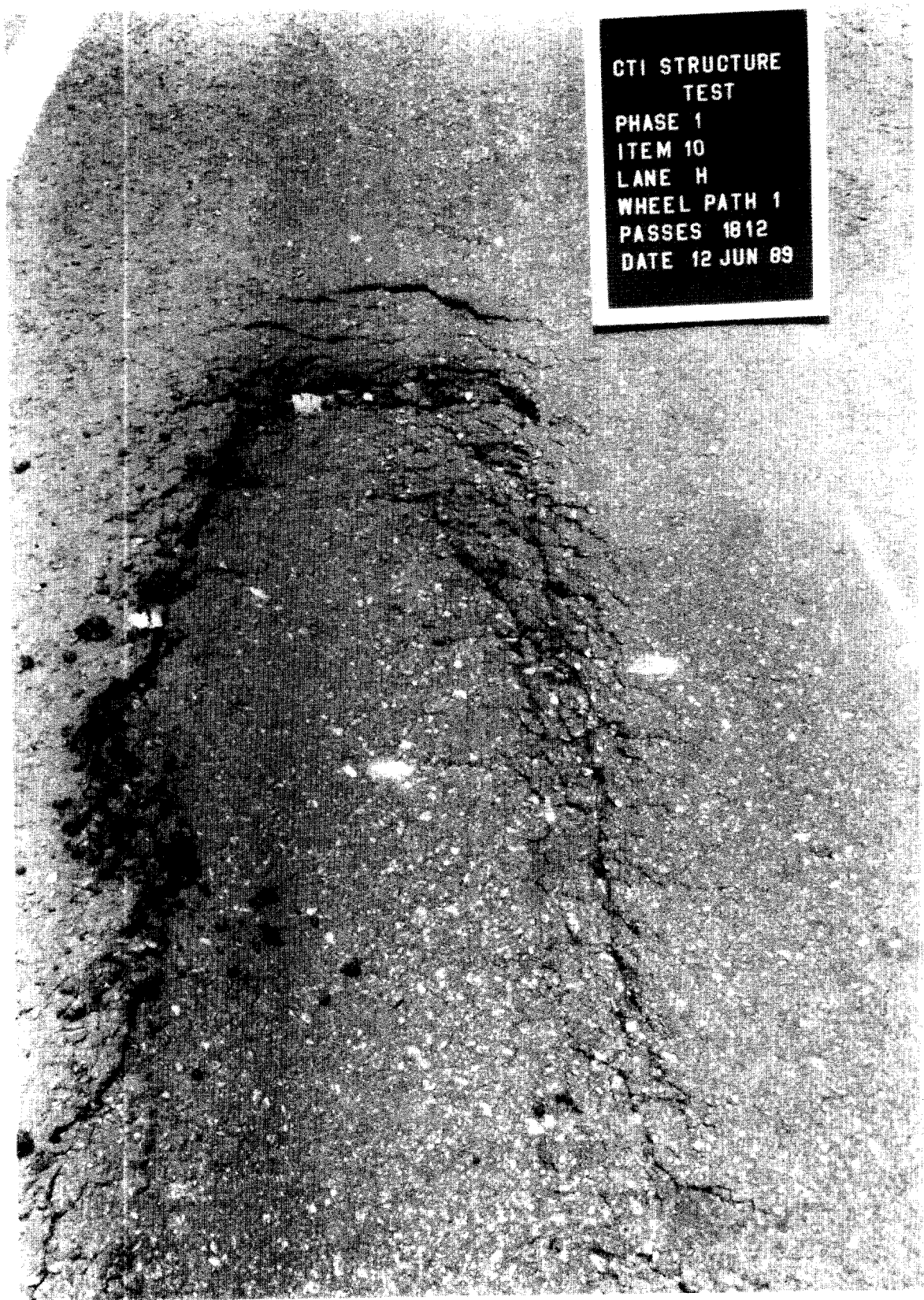
Photo 31 Item 10. wheel path 1. high-severity shoving after 1,812 passes
