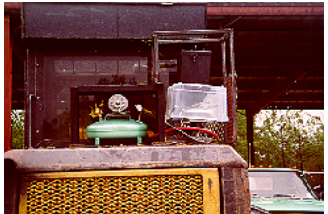
Figure 3—DC-powered air compressor and reservoir.
