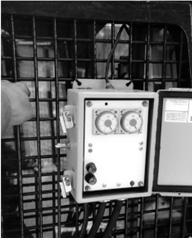
Figure 5—Timers in electrical control box for adjusting amount of air and dry powder delivered to nozzle.
